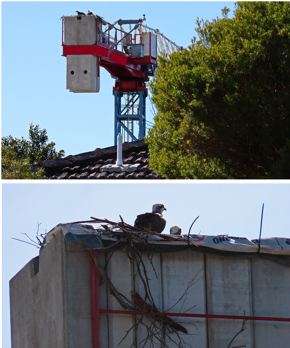
Figure 1. The Eastern Osprey nest situated on top of a construction-tower crane. Photos: Matthew Mo
